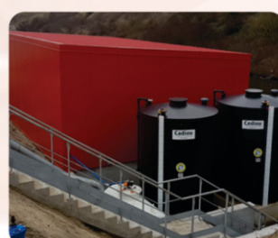
Fire water and foam Pump station
