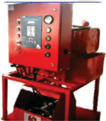
Fire Pumps Control panel
