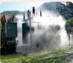
Transformer Fire Protection
