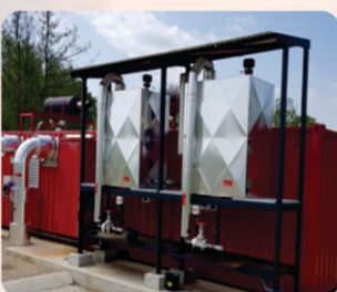
Fire water Pump station in container
