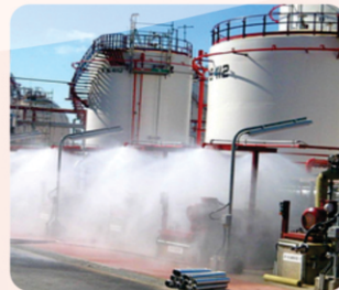
Pump house water spray
