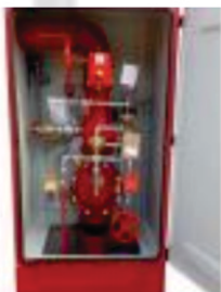
Deluge Preaction Sprinkler
