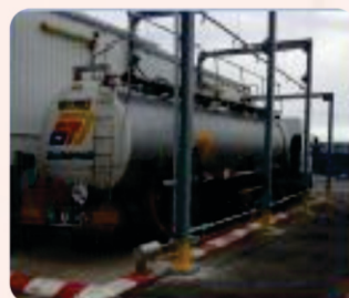
Deluge Preaction Sprinkler
